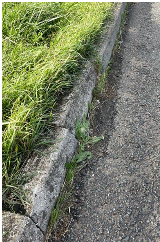
Figure 17: Photo of Potton Road- dislodged kerbs
