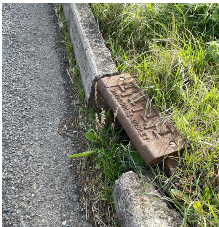
Figure 18: Photo of Potton Road – Dislodged Gully outlet
