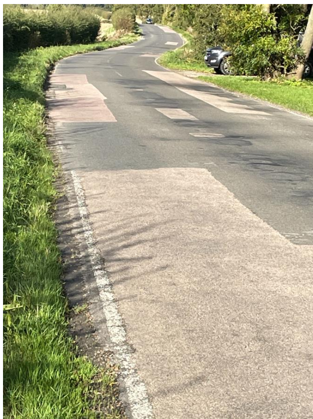
Figure 4: General View of Toseland Road showing repeated edge repairs
