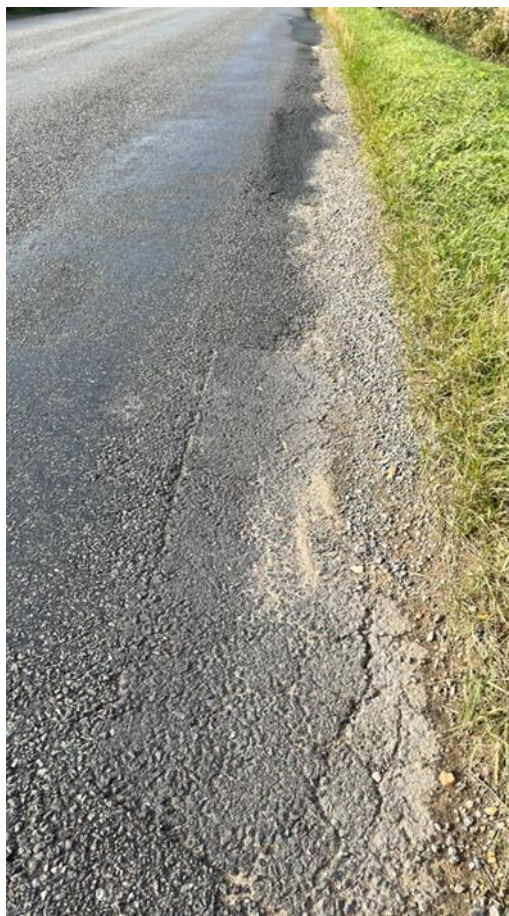
Figure 16: Photo of Potton Road, Edge failures and repairs
