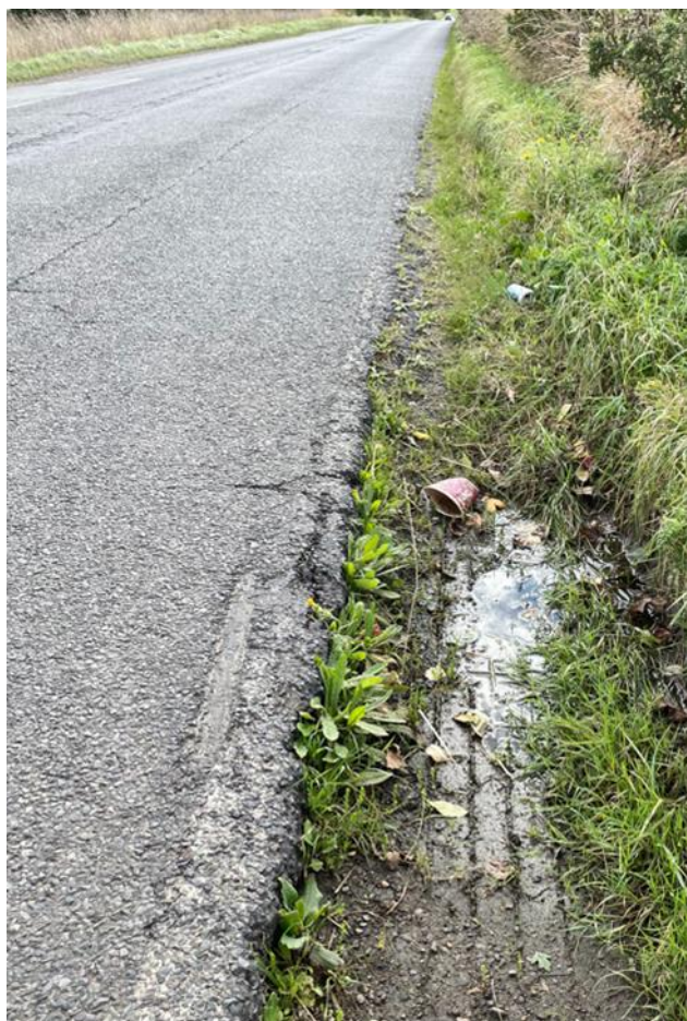
Figure 6: Toseland Road – vehicles running on verge
