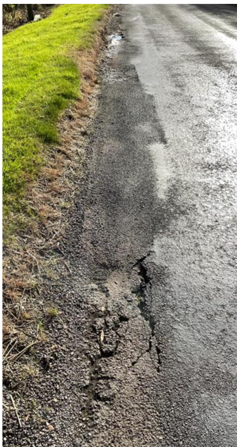
Figure 19: Photo of Potton Road – edge failures and repairs
