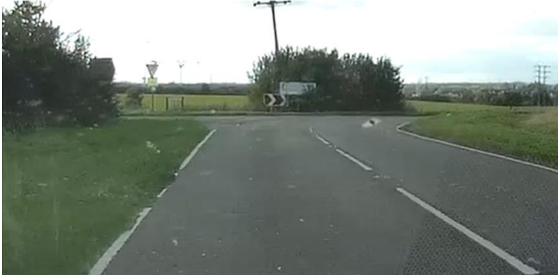
Figure 15: Photo of B1046, edge damage
