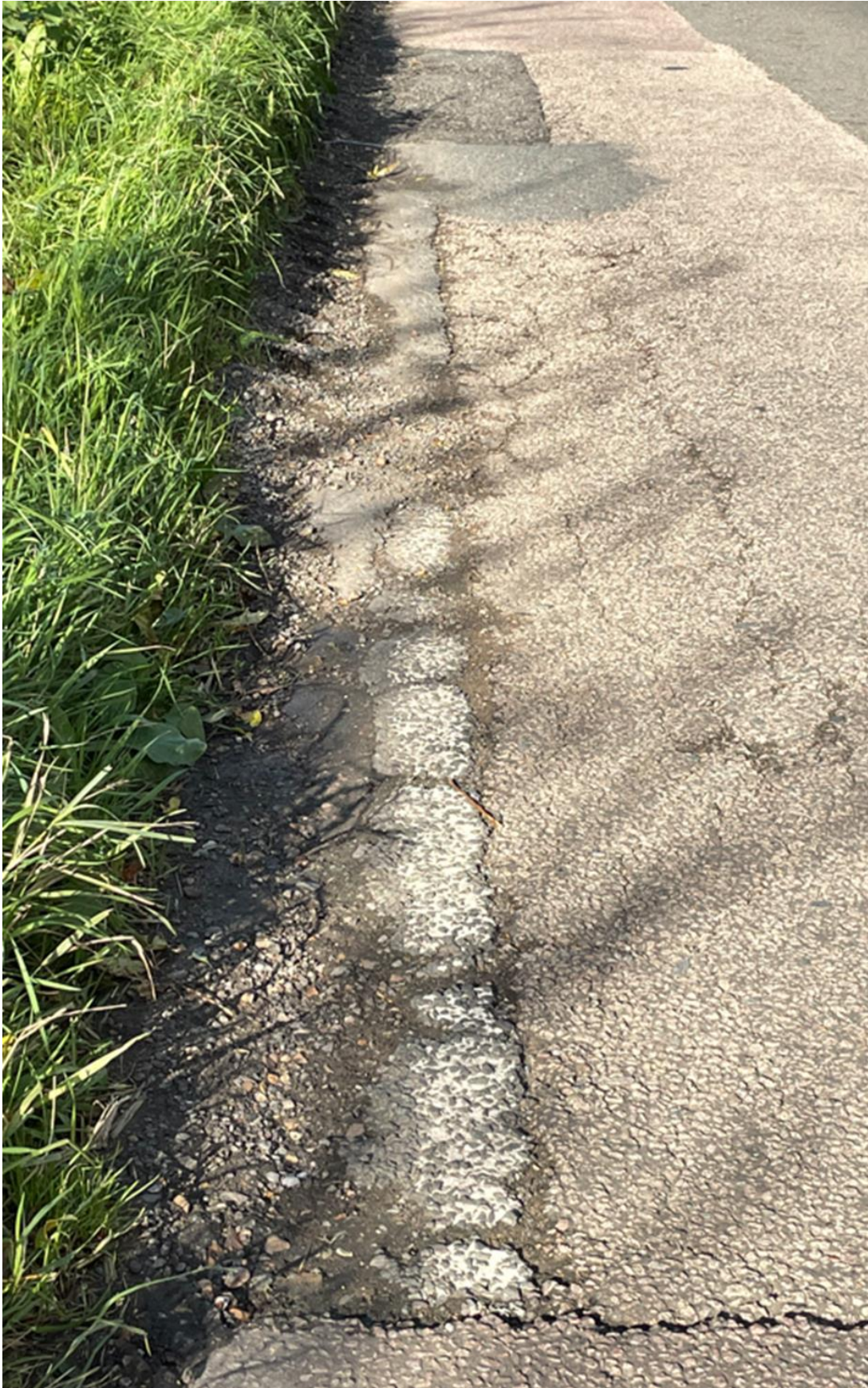
Figure 8: Toseland Road- Previous edge repairs failing again
