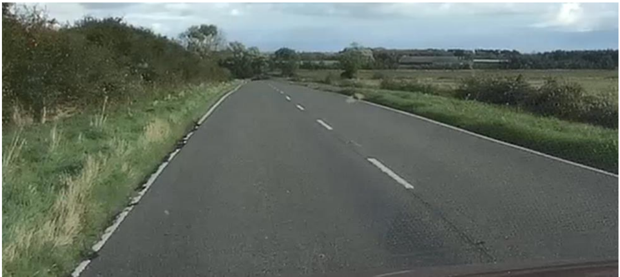
Figure 14: Photo of B1046, edge damage on 6m section
