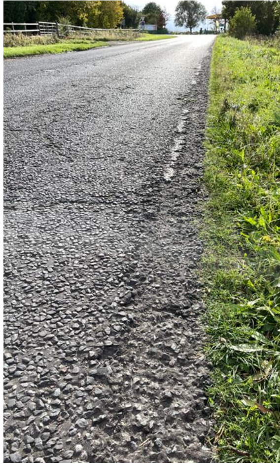
Figure 5: Toseland Road: typical edge condition
