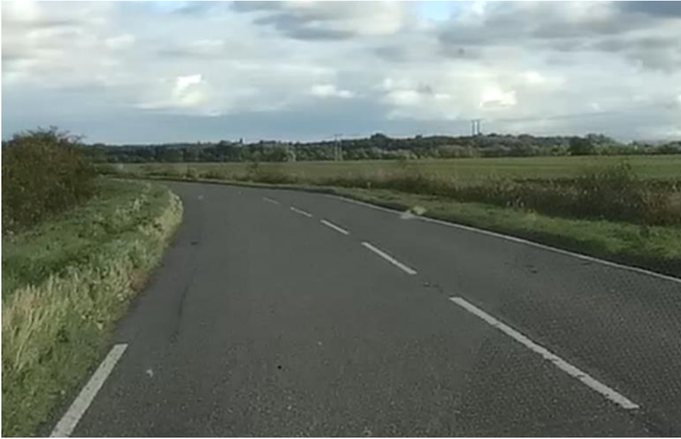
Figure 13: Photo of B1046, length to be diverted, edge repairs on 6m section
